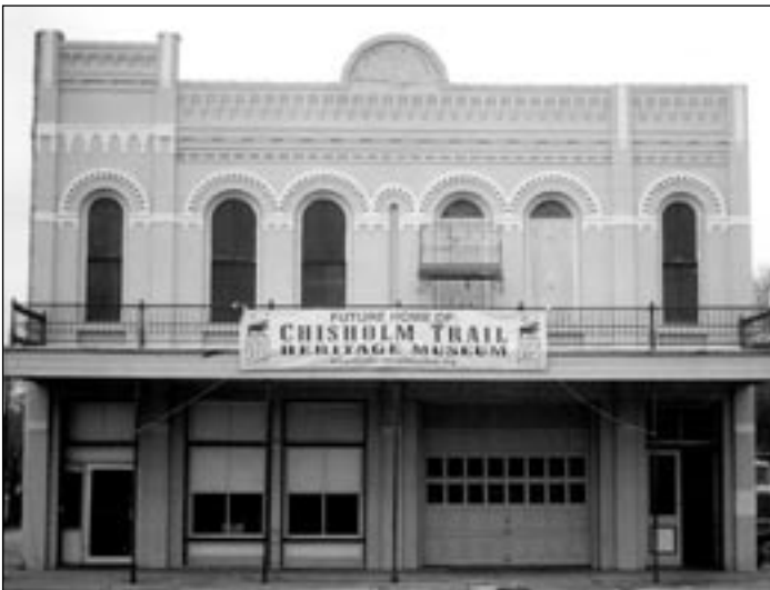
Before: inappropriate alterations, such as the garage door
