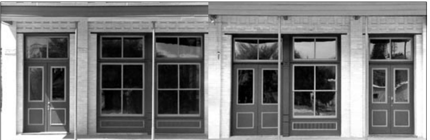
After: Removal of entrance aluminum door and restoration of doors and window in front
